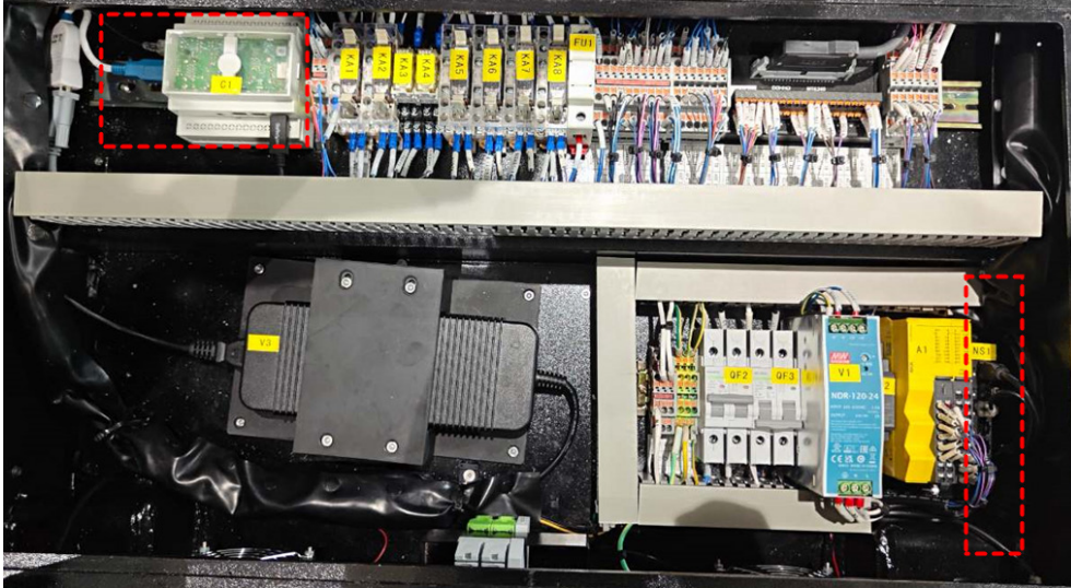
Figure 5.75 Check network cables
